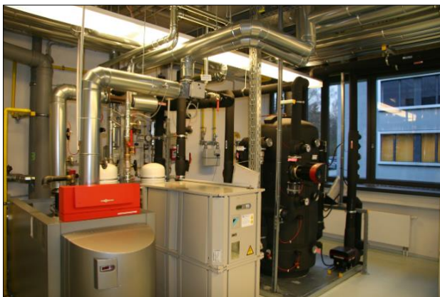
Fig. 1: Test bench (from left to right): gas-condensing boiler, compression chiller, thermal storage
